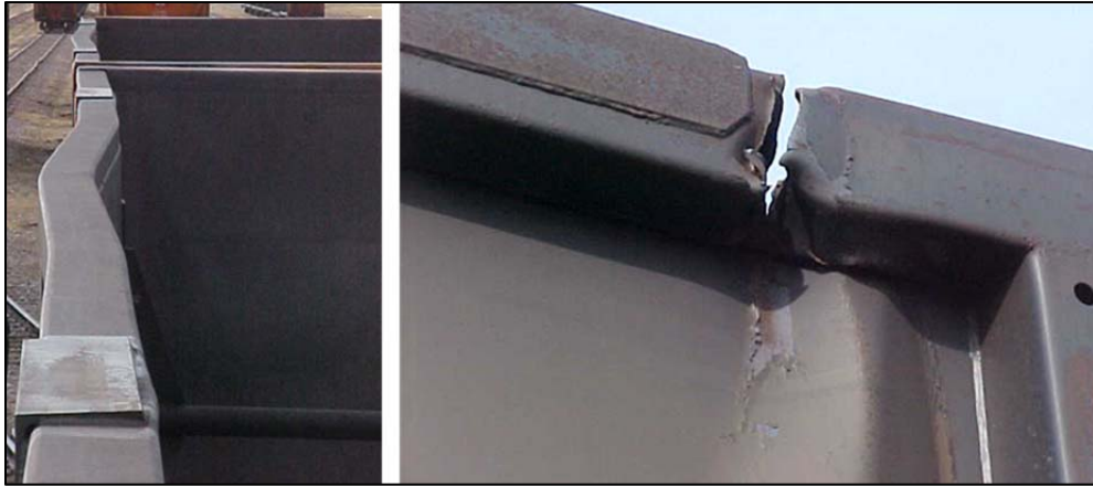
Figure 11: Photographs of buckled top chord and associated fracture
