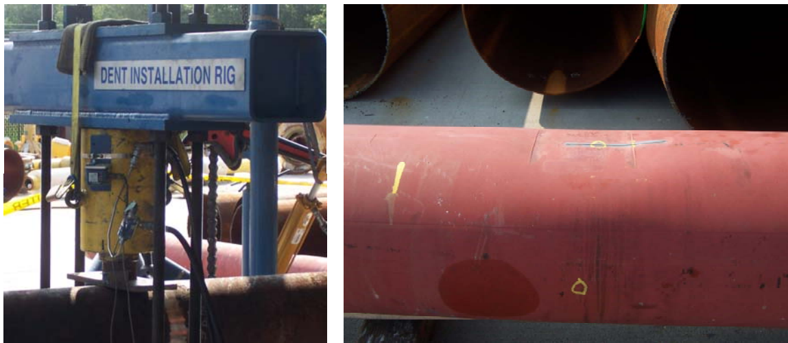
Figure 1 – Efforts associated with dent work including final dent depth
