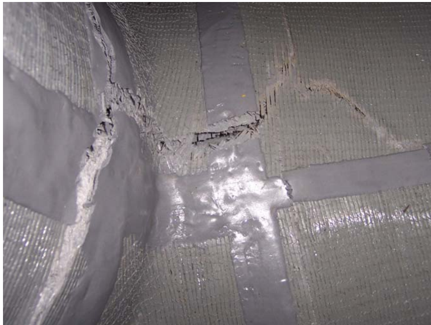
Figure 7 - Crack in composite material in crotch region of branch connection
