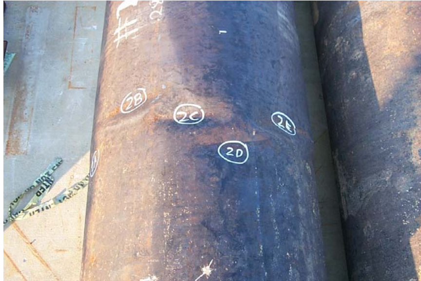
Figure 1 – Photo of 36-inch diameter pipe with 2% wrinkles
