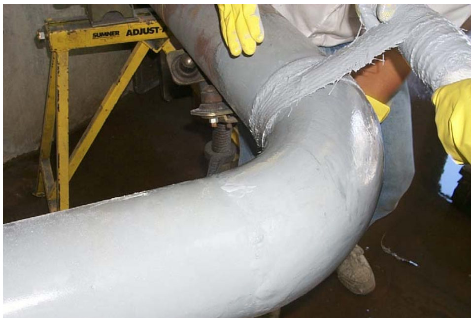
Figure 5 – Repair of pipe elbow fitting using System B 6-in standard wall elbow with 50% corrosion Unrepaired burst pressure of 4,532 psi • Repaired burst pressure of 6,780 psi
