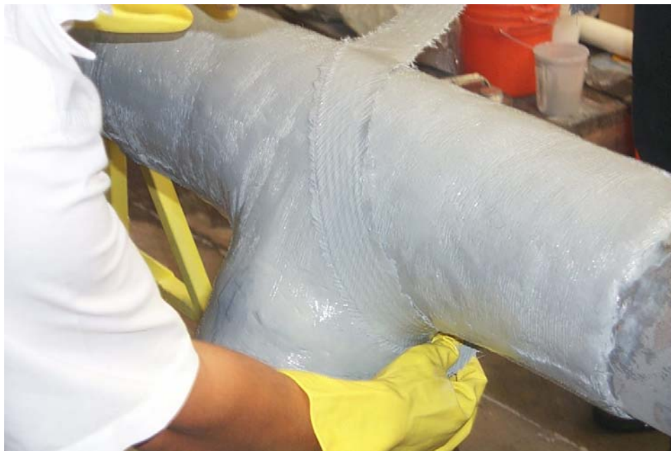
Figure 6 – Repair of pipe tee fitting using System B 6-in standard wall tee with 50% corrosion Unrepaired burst pressure of 6,546 psi • Repaired burst pressure of 7,500 psi
